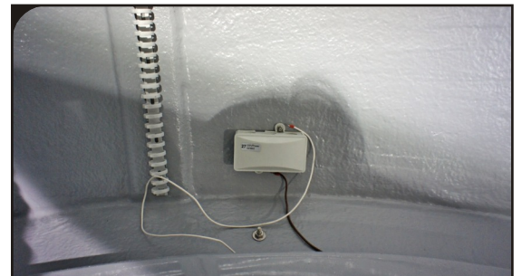
Shutter electric connection box
